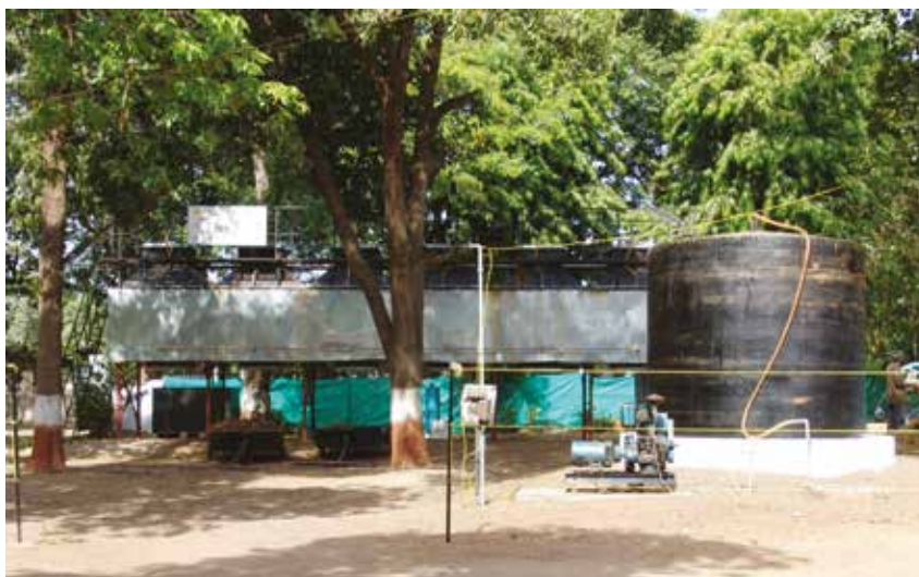
Picture 1: Overview of the pilot plant installed at SPRERI
